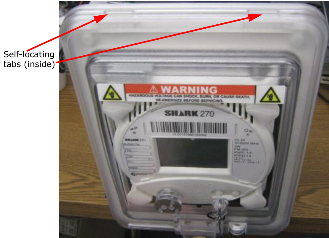
Figure 5.21: Reinstalling the Bezel
