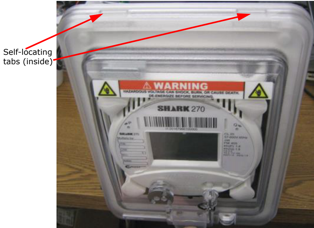
Figure 8.38: Reinstalling the Bezel
