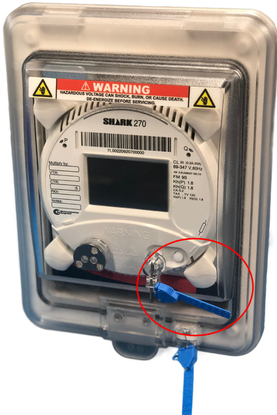
5.25: Sealing the Reset Lever - Switchboard Case Meter
